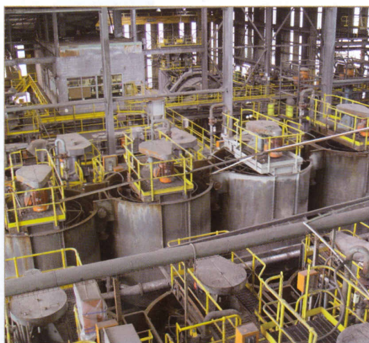
▲ Part of the plant's circuit.
