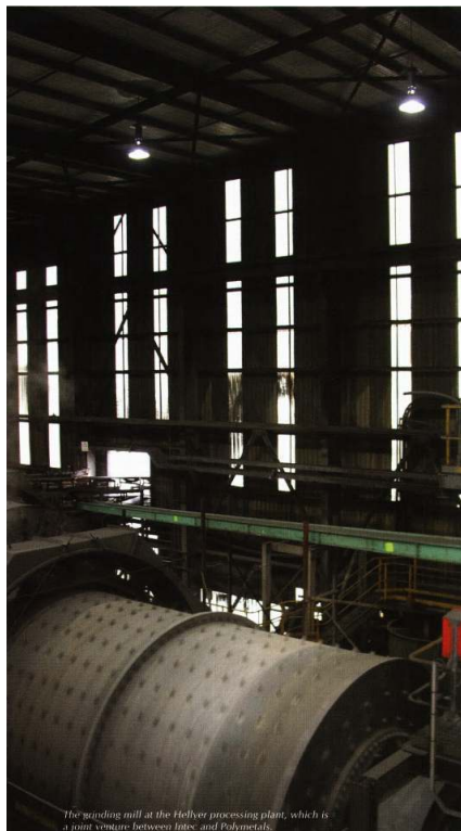
The grinding mill at the Hellyer processing plant, which is a joint venture between Intec and Polymetals.
